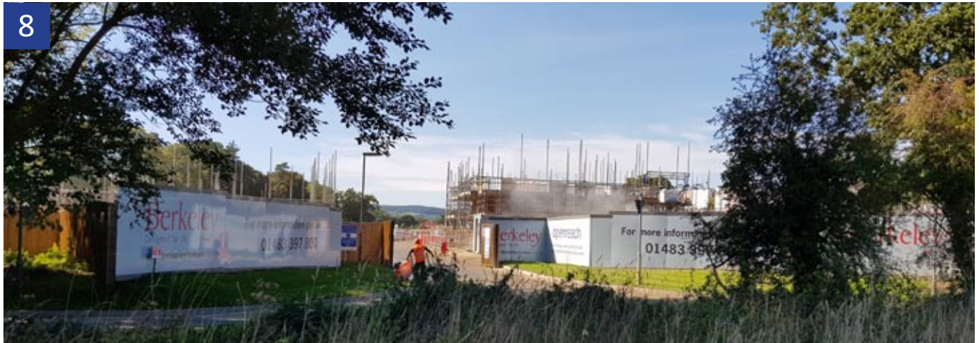
Context Photograph - Entrance to Berkeley Homes site opposite proposal site, west of Knowle Lane
